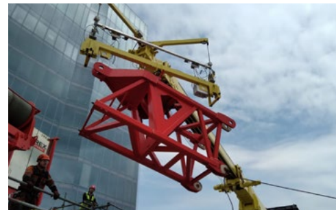
The ability to lift up to 2 t makes BMU a perfect choice for Terex CDK 100-16 crane dismantle.
